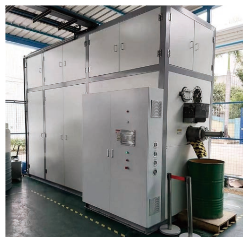
Tail Water Evaporation Equipment No. 1
