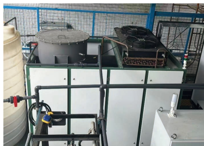
Tail Water Evaporation Equipment No. 2
