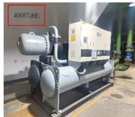
Update of 400RT chiller in the HVAC room on the 1st floor
